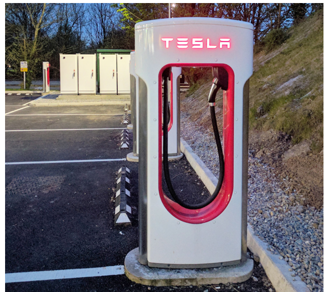
Fig. 26 | Electric vehicle charging point
